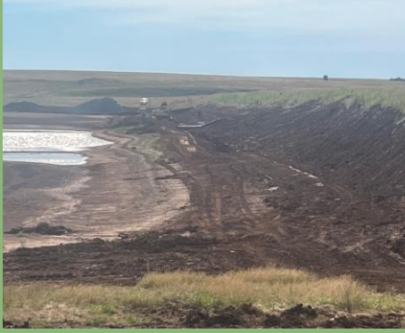
Lower Red Rock watershed 13 was drained and repaired due to front slope damage. 1,462 tons of riprap were used to protect 700 feet of slope.
