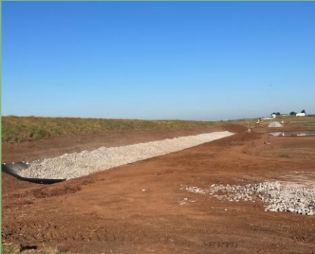
1,546 tons of riprap was required to protect 1,340 feet of front slope on Upper Black Bear watershed site 2 in Noble County.
