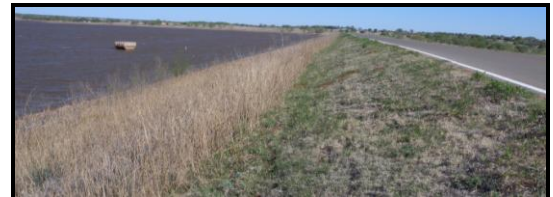
Upper Elk Creek Watershed Dam No. 22 provides flood control and recreational areas.
