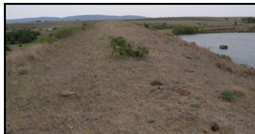
Rainy Mountain Watershed Dam No. 10, one of 29 flood control dams in the watershed project.
