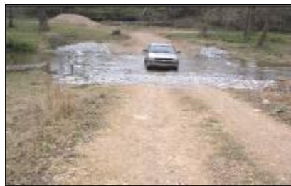
This stream crossing was stabilized with re-engineering and rock to prevent further erosion.
